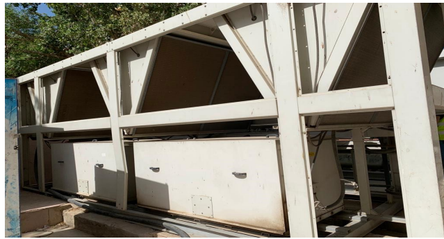
Figure 1 The Existing Chill
